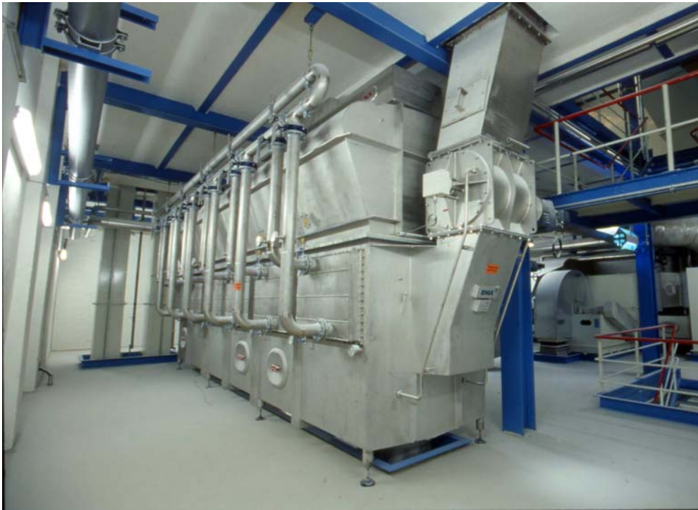
Fig. 3: Horizontal fluidized bed cooler with integrated cooling blocks
