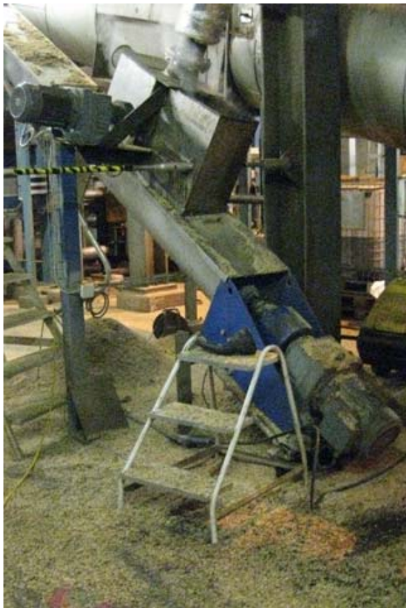
Fig. 12, first pulp discharged trough the outlet pipe.
