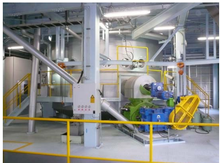
Fig. 3, steam dryer in operation.
