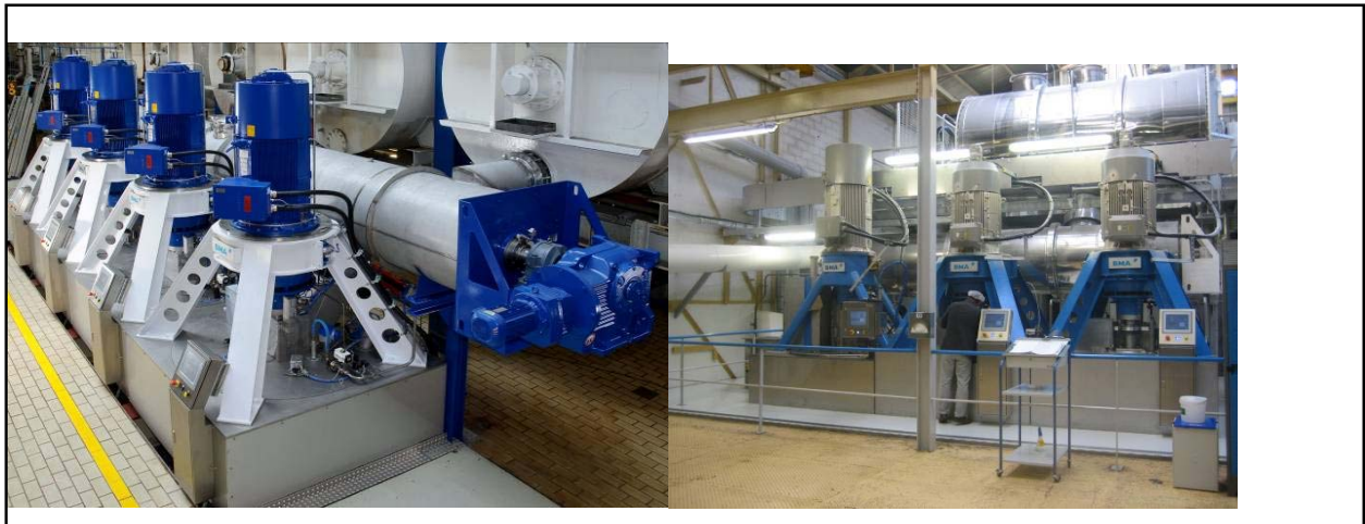
Fig. 12: New centrifugal station equipped with four E1810 Südzucker's Plattling sugar factory (Germany)
