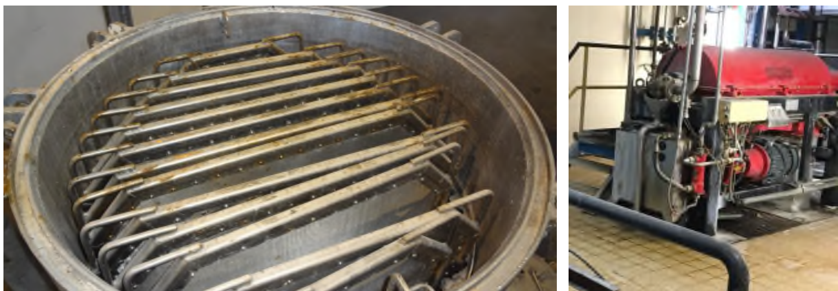
Figure 1: Left: existing plate type precoat filters / Right: Slurry decanter
