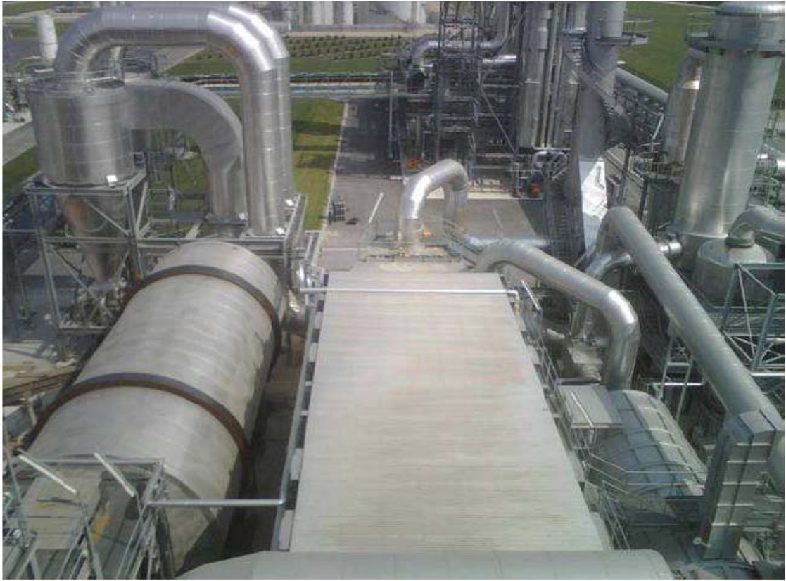
3 PASS DRYER -----Heat Exchanger-----Furnace
